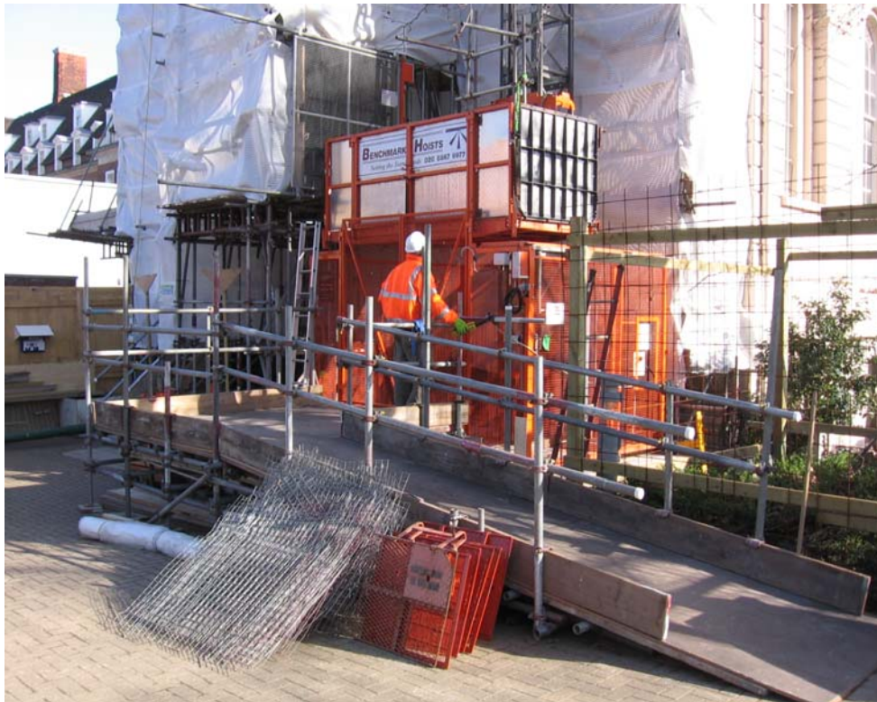
Photo 2 - M15/32 with C door in cage & enclosure for side loading at base level
