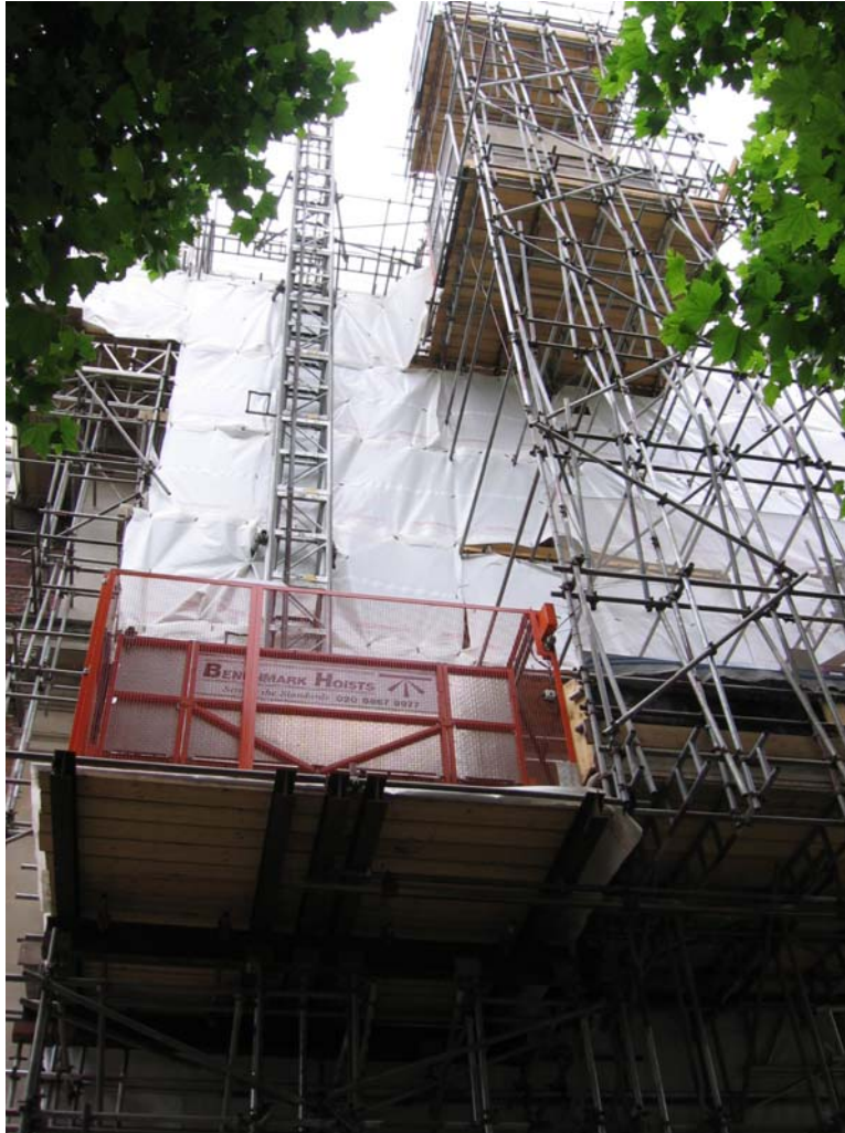
Photo 2 - Gantry mounted Goods Hoist M15/32 & 1.5T Beam Hoist
