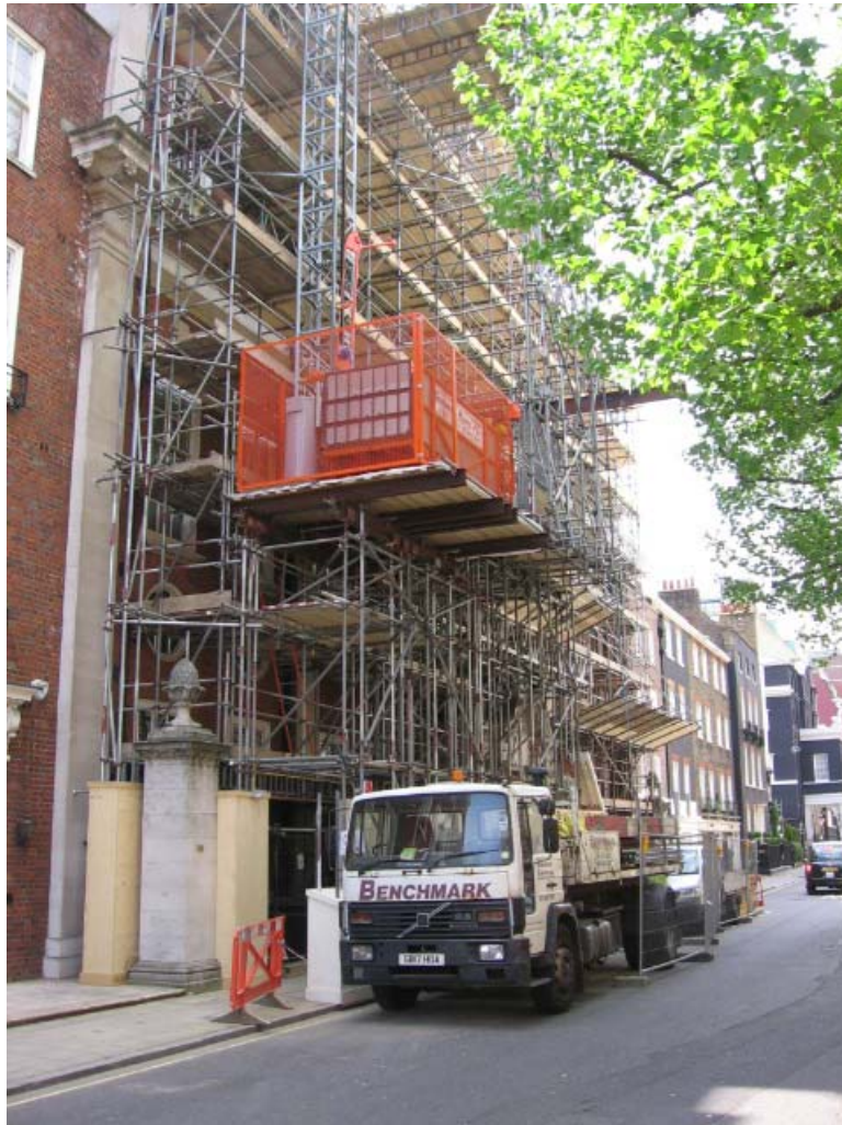
Photo 1 - Gantry mounted Goods Hoist M15/32 & 1.5T Beam Hoist
