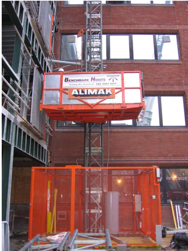
Photo 1 - M15/32 Goods Hoist Multibuild New Premier Lodge Hanger Lane
