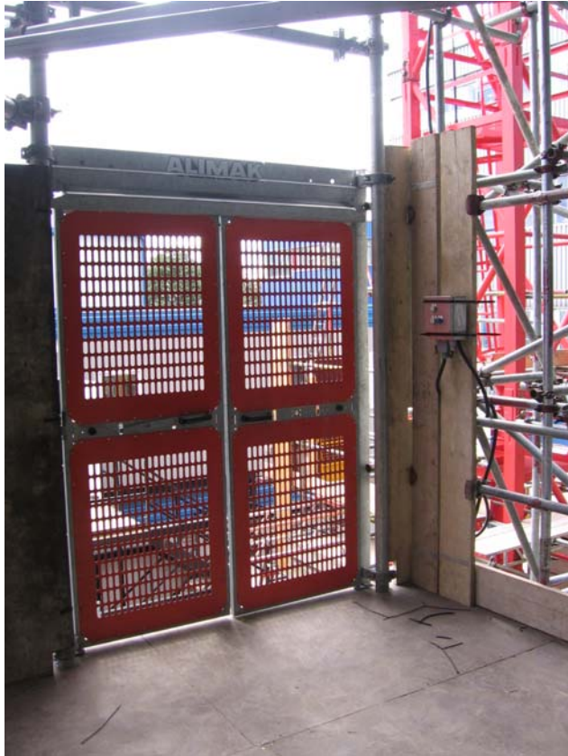
Photo 3 - Landing Level showing push button call station for driverless operation
