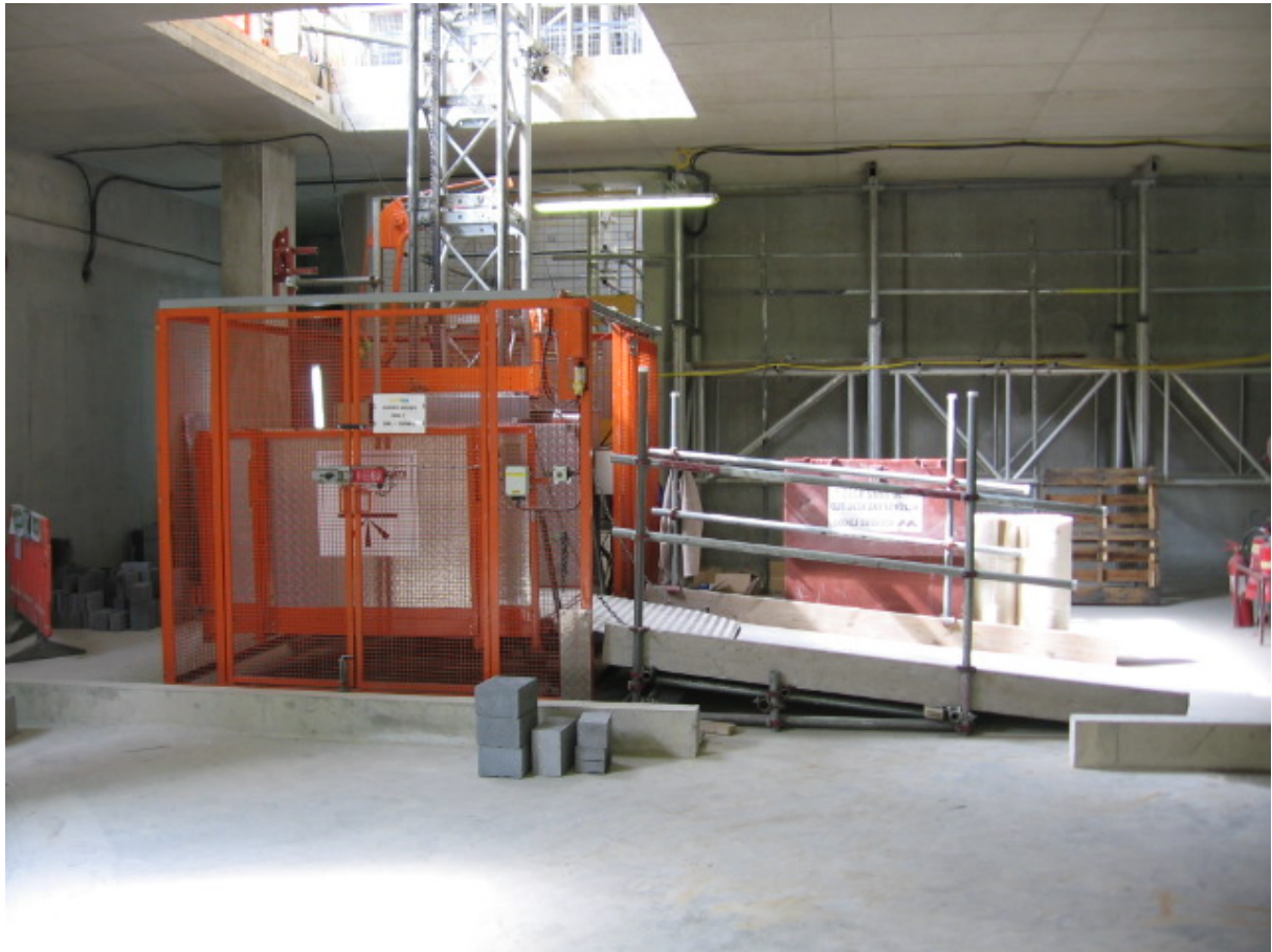
Photo 1 – Basement Goods Hoist M12/20 serving ground to basement level
