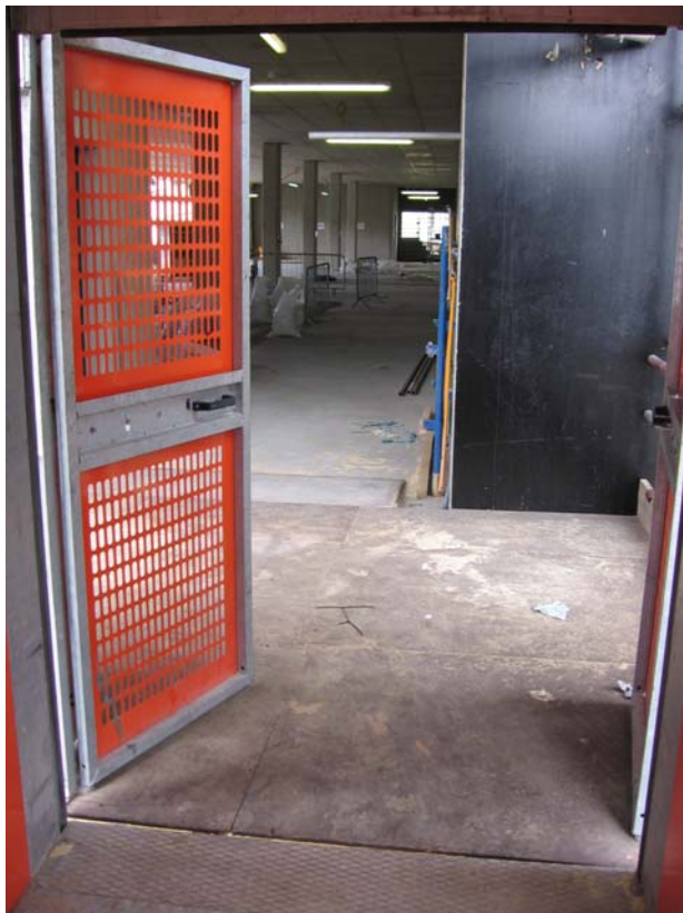
Photo 4 - shows scaffold landing designed for maximum Hoist loadings - flush with Hoist cage floor
