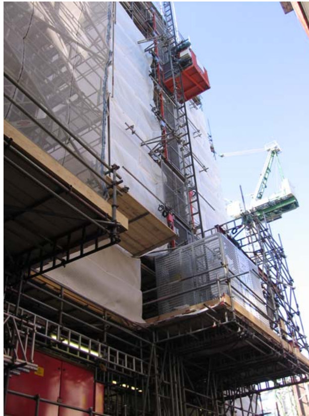
Photo 1 - Gantry mounted M700 Goods Hoist & 1T Beam Hoist
