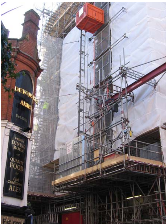
Photo 3 - M700 Goods Hoist & 1T Beam Hoist
